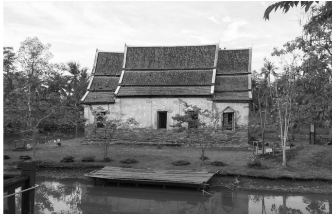
Figure 1 : Ubosot (chapel) at Wat Muen Wai is made of bricks and mortars with base of the chapel is sagged in shape as a junk
